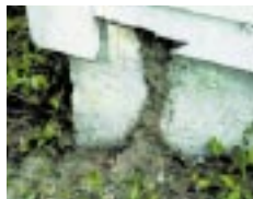
PHOTO 1: Subterranean termites build shelter tubes or mud tubes that serve as “climate controlled” access routes to a building. [Photo: Louisiana State University, Agricultural Center]
